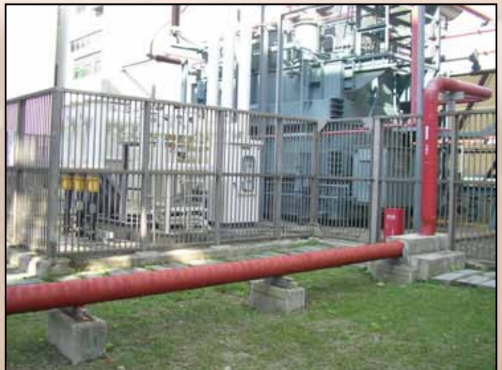
Fire Water Lines
