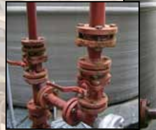
Highly corrosive environment
