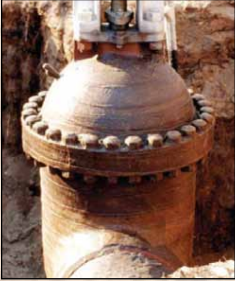
Protection of large valve
