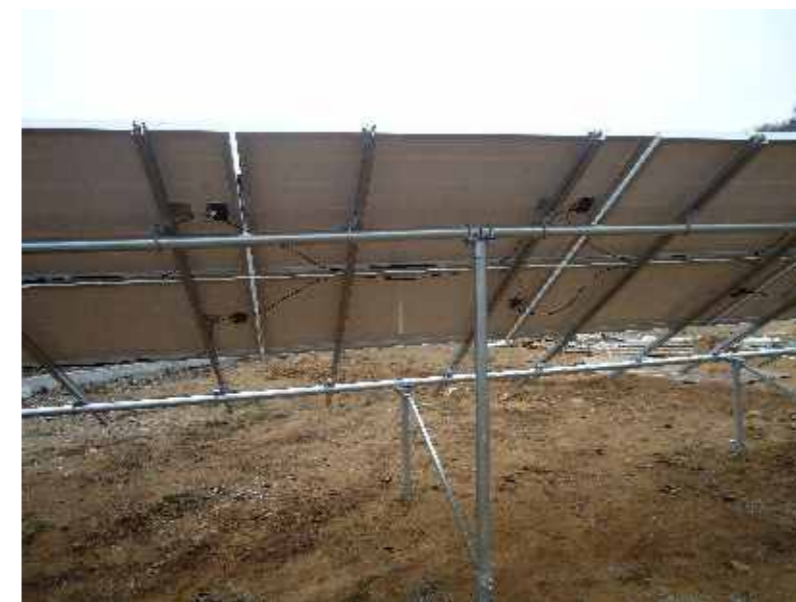
Grace Solar Project in Greece
