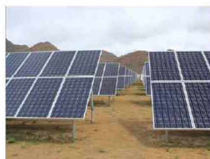
Solar Power Systems
